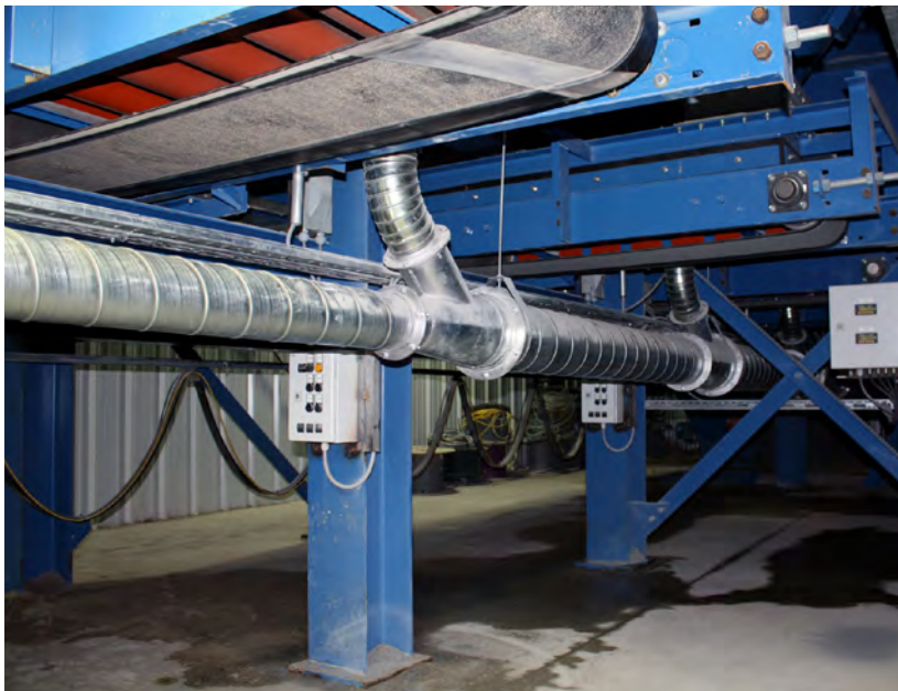
Fugitive silica dust, generated as material is poured into storage silos, is captured at the source and conveyed to an outdoor dust collector through this ductwork system.
