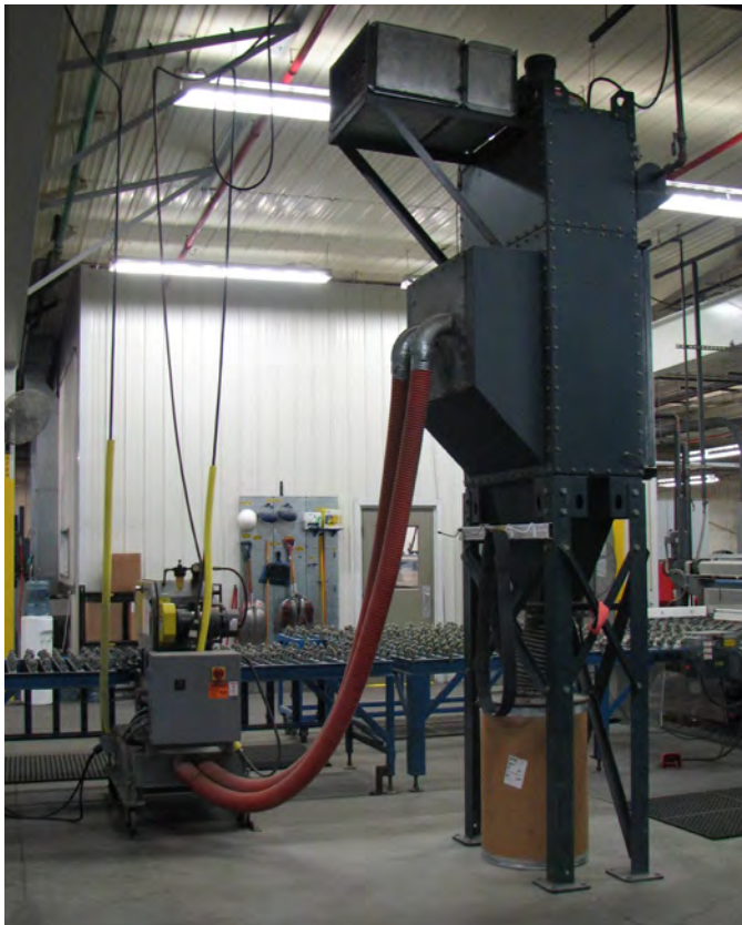
In a glass fabrication shop, high-speed silicon carbide belts are used to take sharp edges off cut glass. A source capture system conveys the silicon carbide and glass dusts directly to the adjacent collector.
